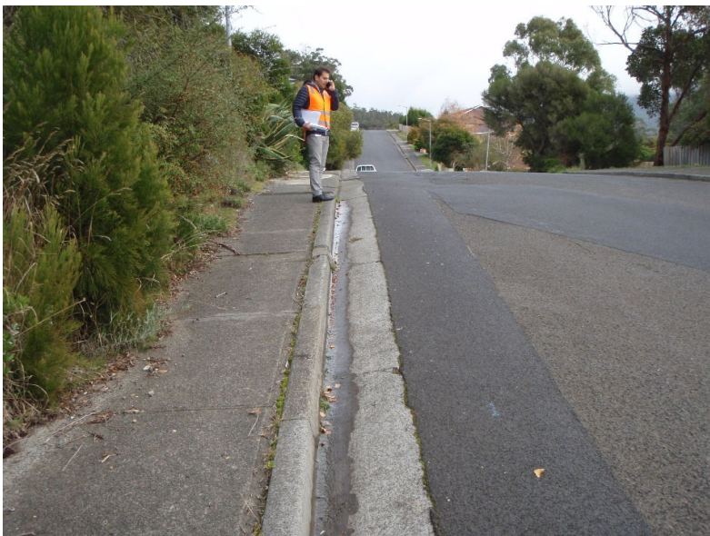
Figure 4 – seepage in the gutter below No 1 Officer Street – see Figure 2 for location.
