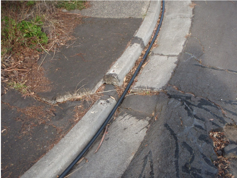
Figure 3 – cracks continuing to open up in the kerb in the cul-de-sac above Hone Rd - see Figure 2 for location.
